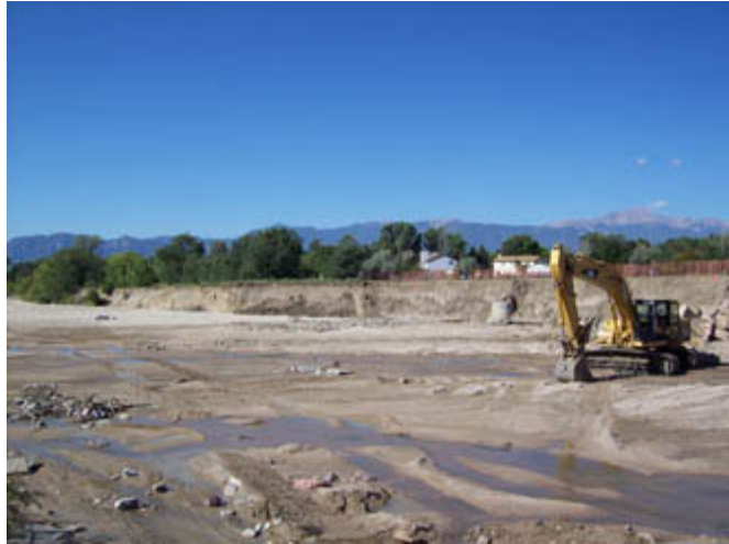
Post-storm work has helped protect wastewater pipes. Photo by Courtesy Colorado Springs Utilities
